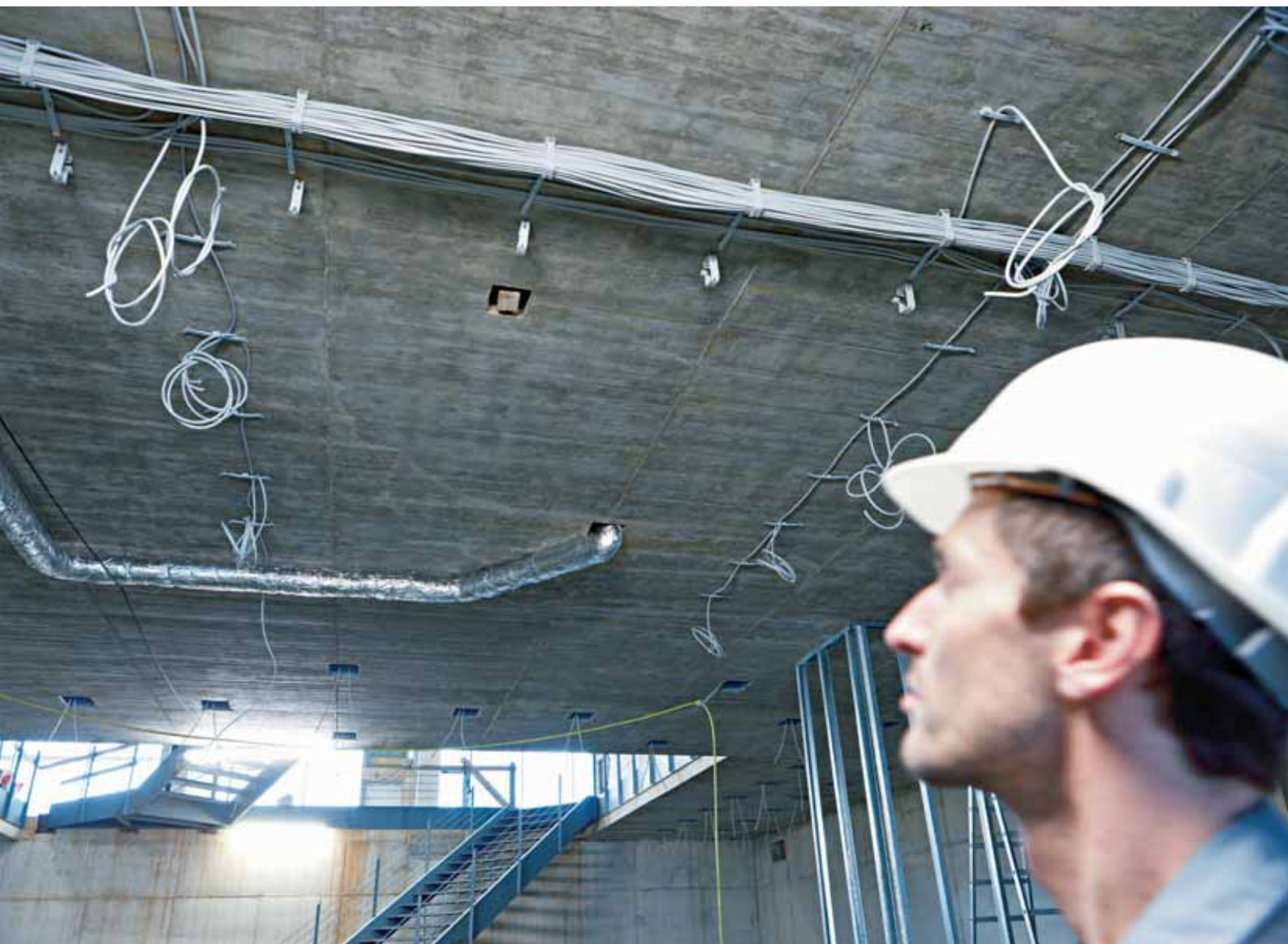
Routing, e.g. with our grouped supports and clamp clips
